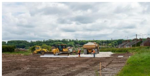
Footprint of embankment stripped of topsoil and stone haul road being installed at South Ferriby
